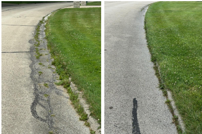
Curbs and gutters which need maintenance: Please remove growth!
